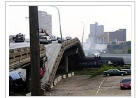
August 1: I-35W Mississippi River bridge collapse.
